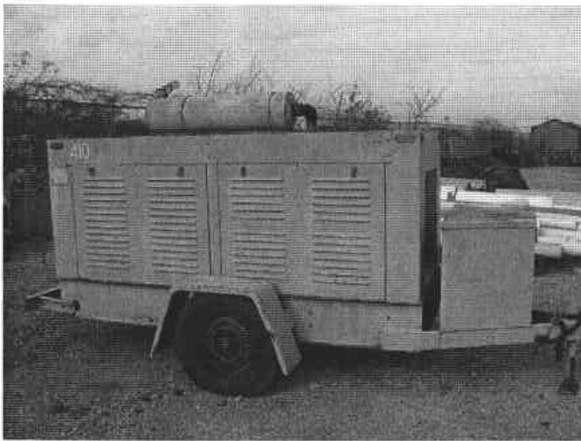
3. Empire Engine Generator Set: 30 KW Model 300 DXW-8E
