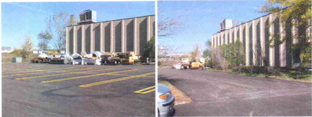
MATERIALS, DEBRIS AND EQUIPMENT AT 423 ST. PAUL
