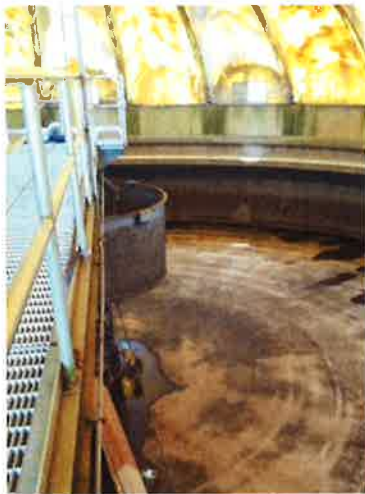
Replaced wear strips and ball bearings on the main gear at clarifier #2.
