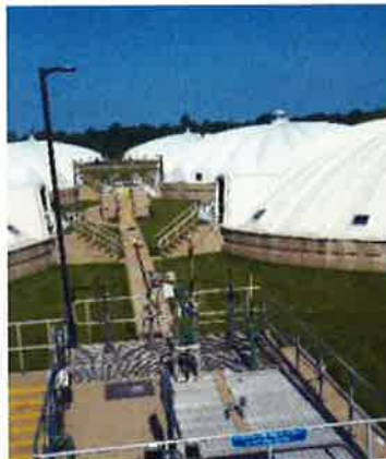
New LED light poles and fixtures.
