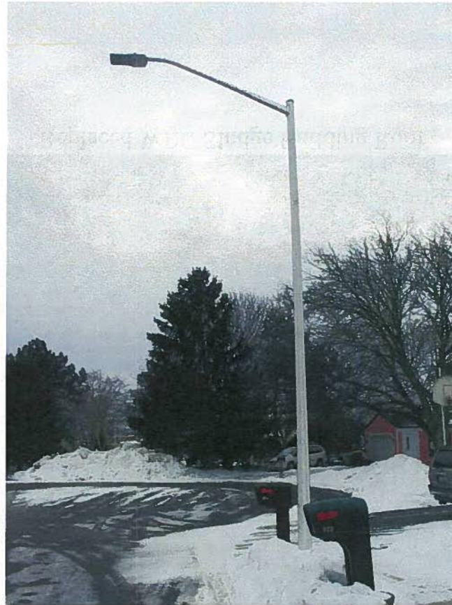
Newly Installed LED Streetlight on Saginaw Court
