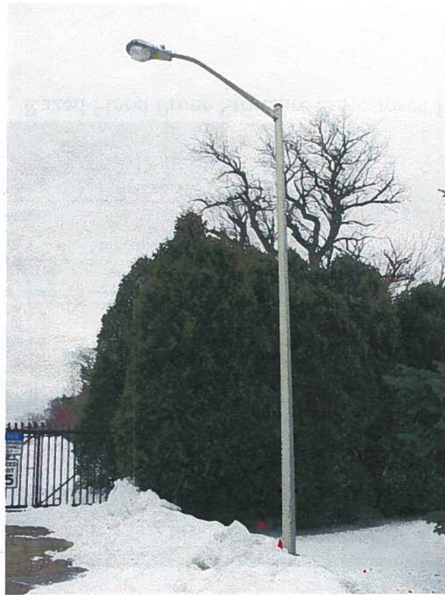
Streetlight at WRC to be Replaced
