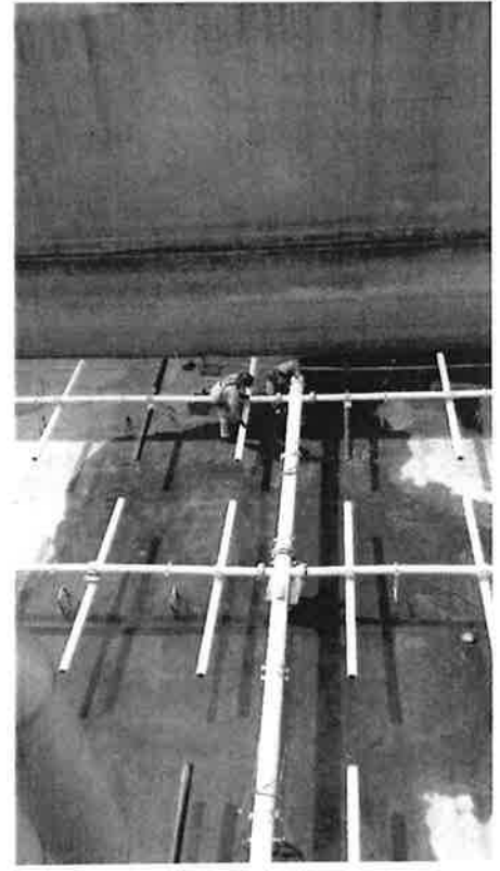
Aeration basin headers for diffusers.
