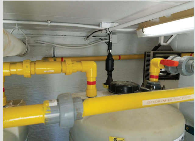
Level sensors installed on sodium hypochlorite and sodium bisulfite chemical tanks.
