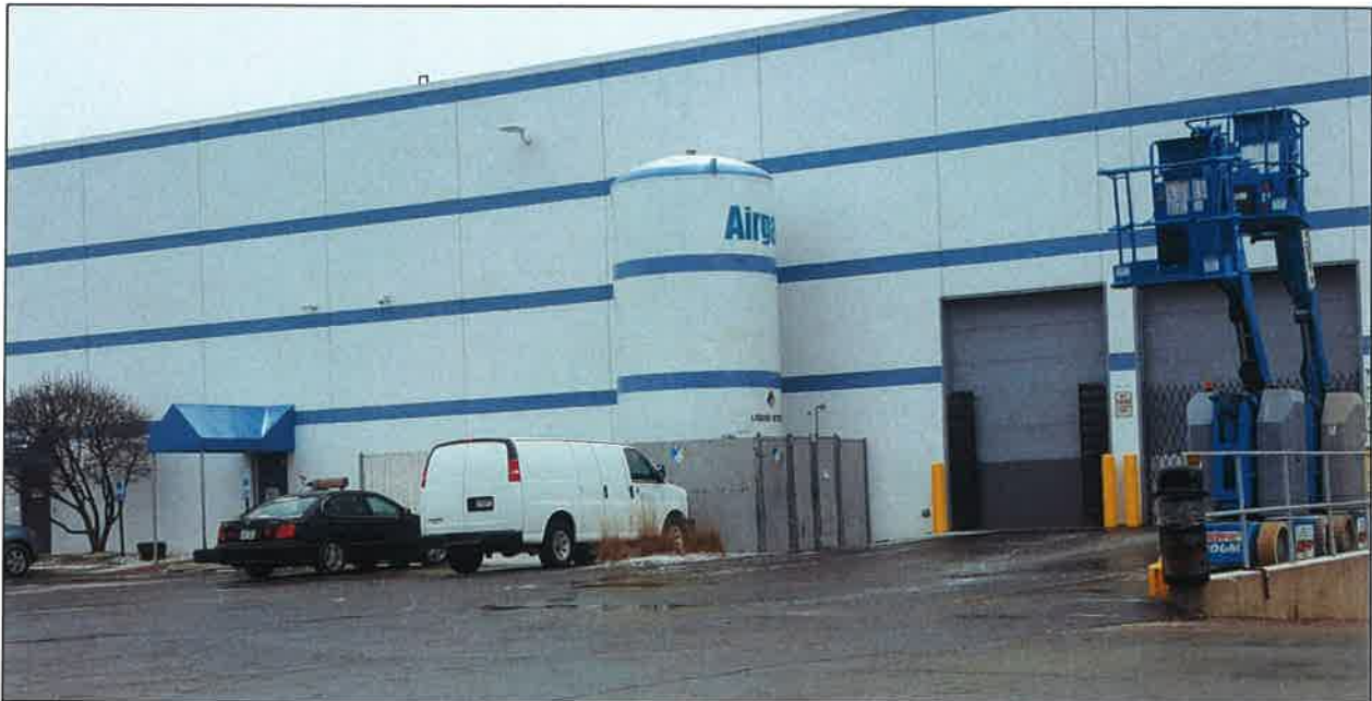
Photo of Existing Tank and Fenced Area on West Side of Property
