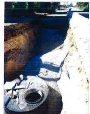
72-inch interceptor was designed in rock adjacent to the I-80 bridge piers.
