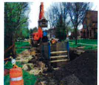
Construction operations had to be well planned and coordinated to reduce impacts to the public.
