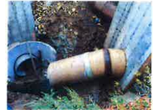
Two junction structures designed to convey existing flows to the new interceptor
