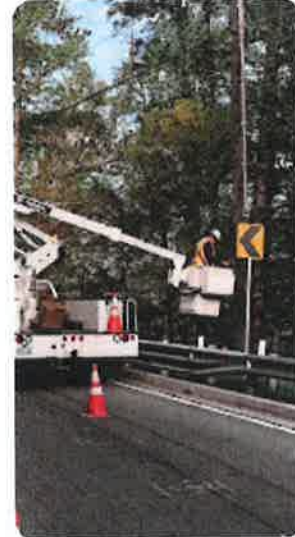
City Foot Traffic Street Electric & existing pole
