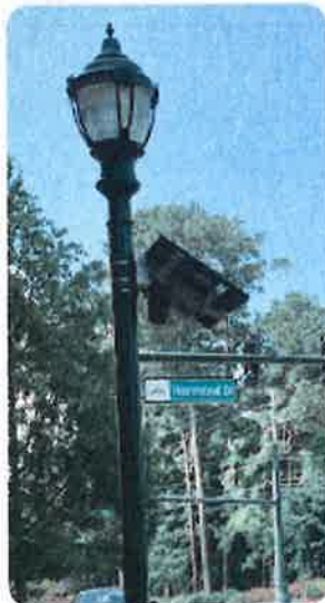
City intersection Solar & existing pole
