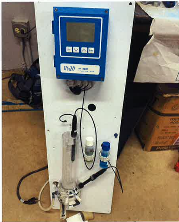
Hach CL17 Chlorine Analyzer SN#9844
