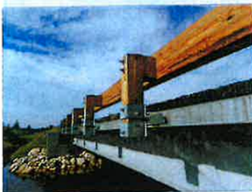
A St. Louis County composite timber and steel bridge features wooden railings.
