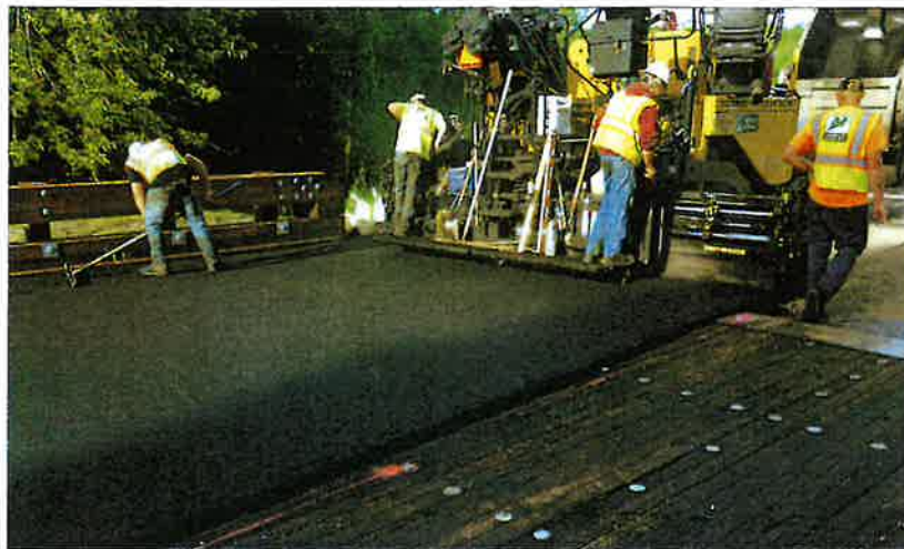
A construction crew in Hennepin County lays asphalt over spike-laminated timber decking for a 2019 bridge in Dayton. Crews would later add a waterproof membrane and an asphalt wearing course.
