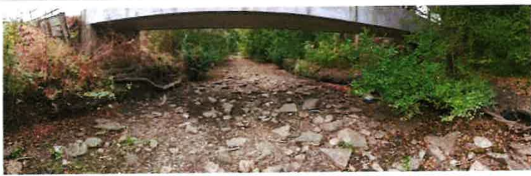
Photo 2 - View of streambed during a dry spell looking north at Library Bridge (October 2017)
