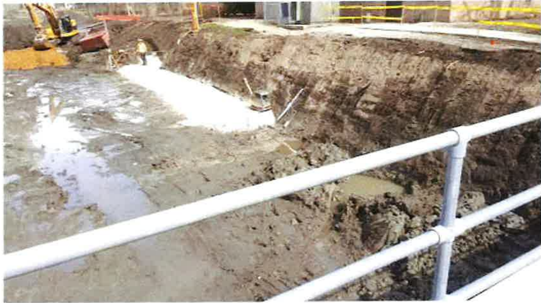
Photo 10 - View of test pits to determine the depth to suitable subgrade for Wall "C" (March 12, 2024)
