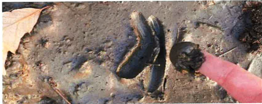
Photo 8 - Peat subgrade beneath Retaining Wall C (March 4, 2024)
