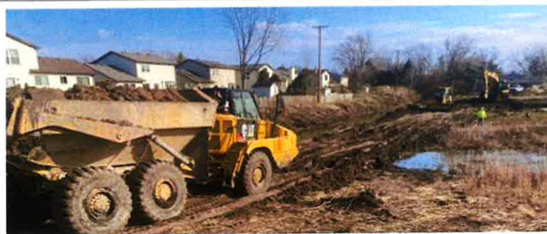
Photo 14 - Hauling suitable material from the south wetland to backfill the streambed (March 28, 2024)
