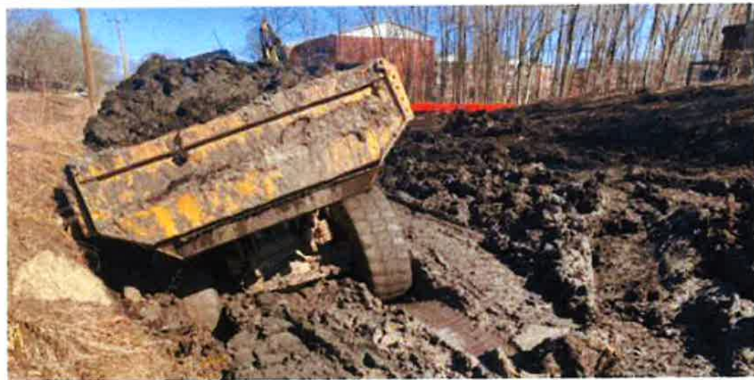
Photo 9 - Unsuitable streambed material impacting construction progress (March 11, 2024)
