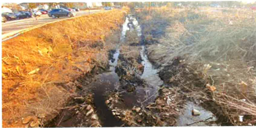
Photo 5 - Ruts in existing streambed caused by tree clearing equipment (February 24, 2024)
