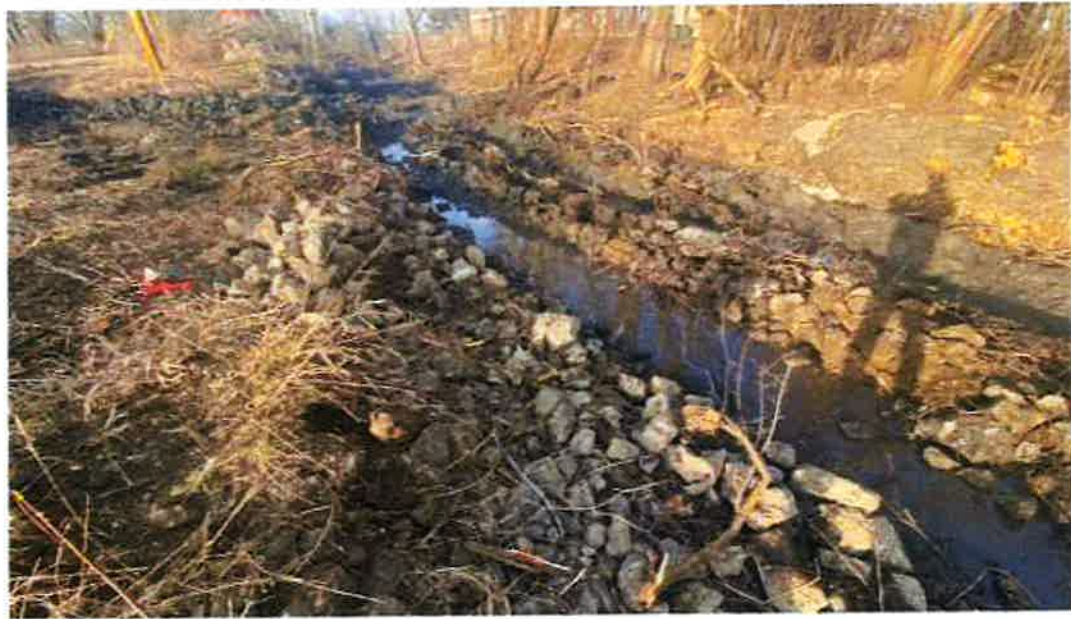
Photo 3 - Ruts in existing streambed caused by tree clearing equipment (February 22, 2024)
