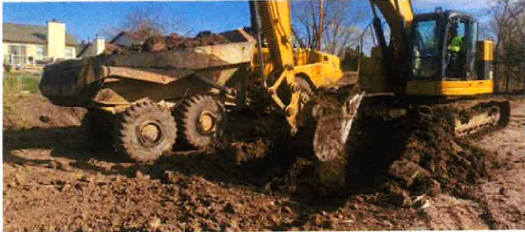
Photo 15 - Excavating suitable material from the proposed wetland area for backfilling the streambed (March 28, 2024)
