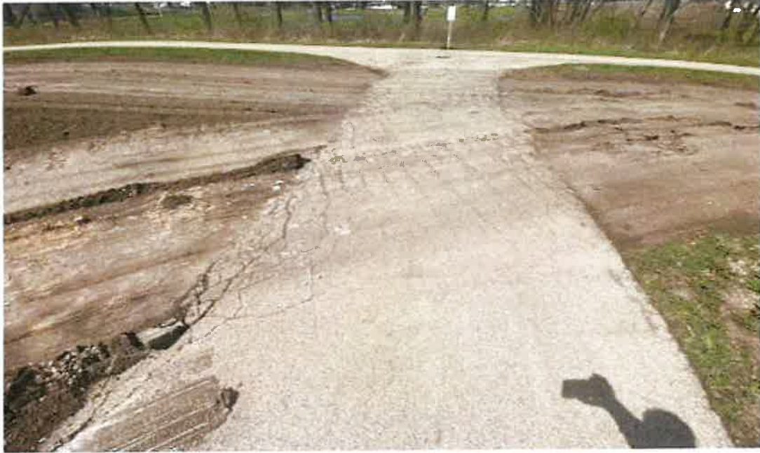
Photo 13 – Looking west at the damaged path near the northwest corner of Mitchell Lakes (04 12 2024)
