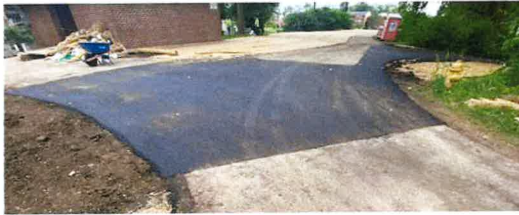
Photo 12 - Looking south at the path repair in front of the well pump house (06/13/24)
