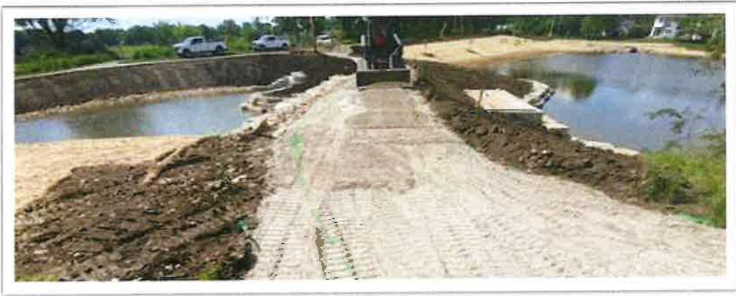
Photo 5 - Looking northwest at the aggregate base being added over the Mitchell Lakes outfall (06/03/24)
