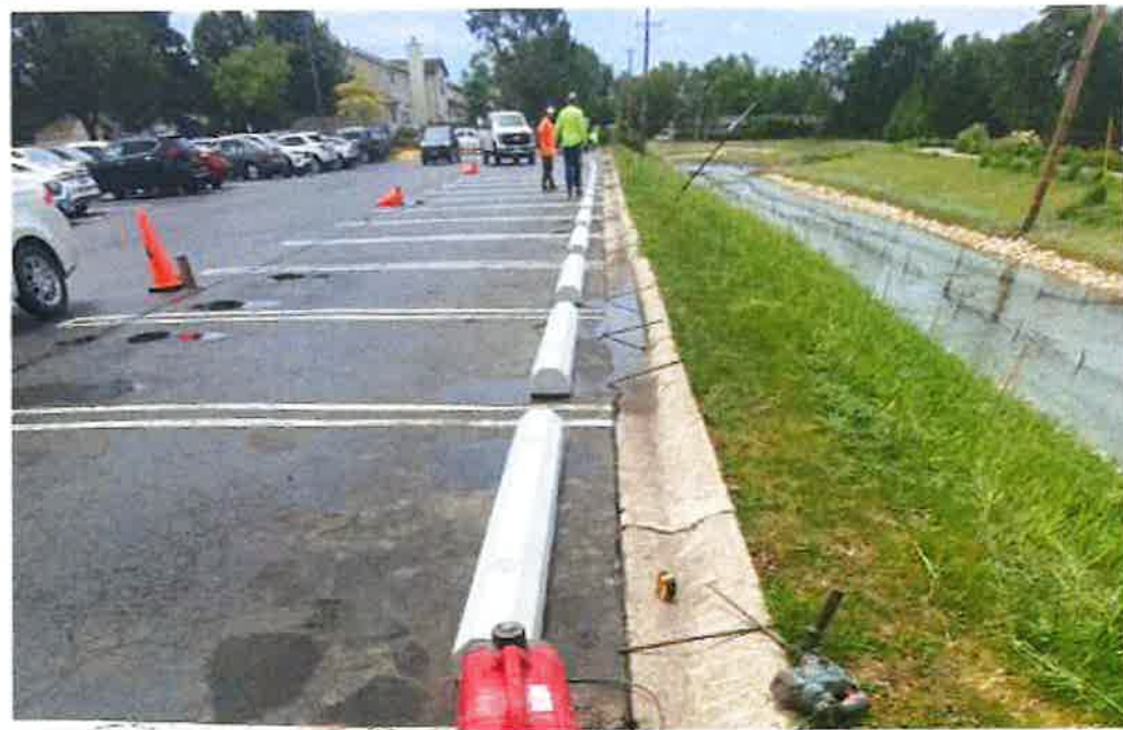
Photo 16 - Looking south at the new wheel stops along along the western edge of the library parking lot (06/25/24)
