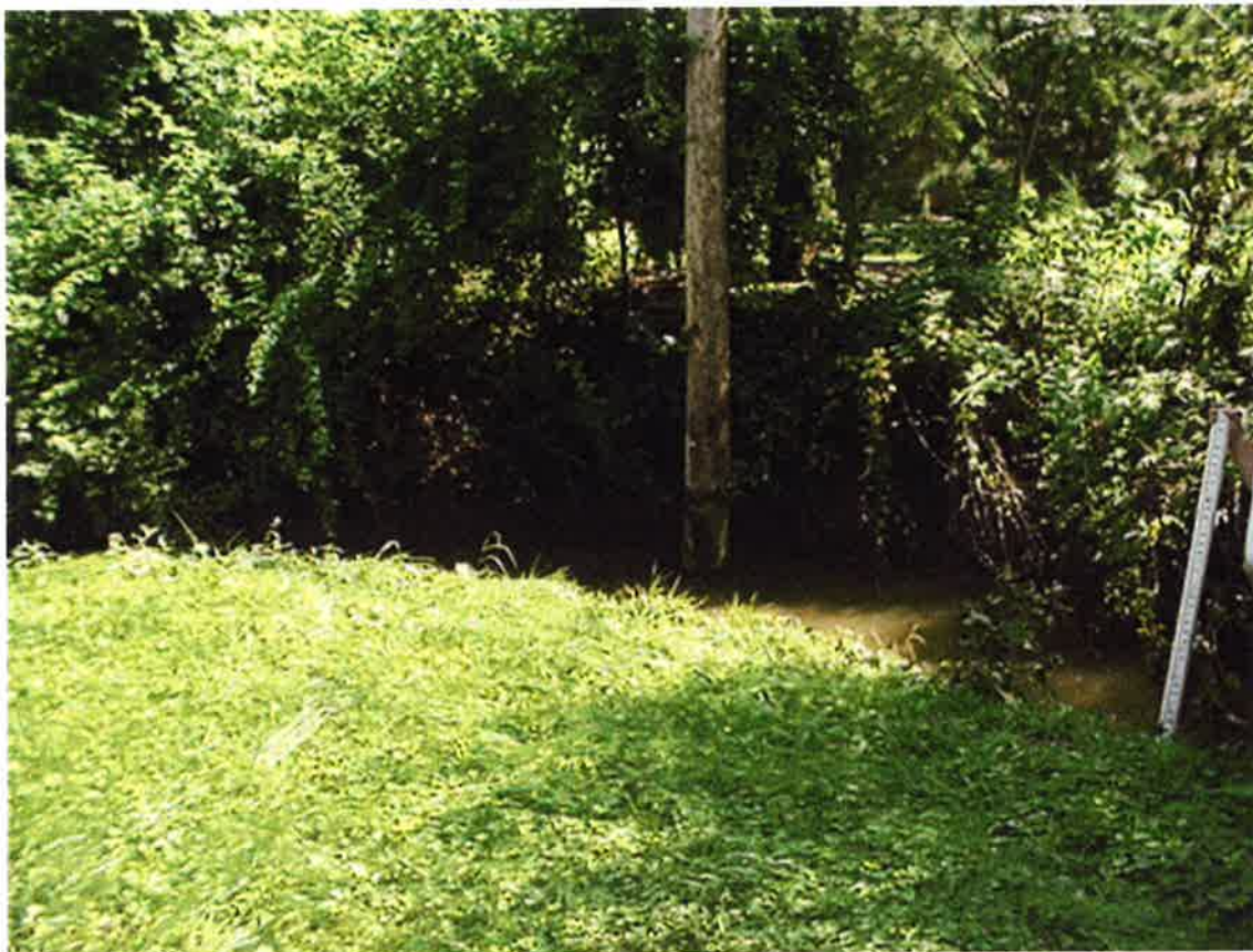
Erosion Around a ComEd Utility Pole
