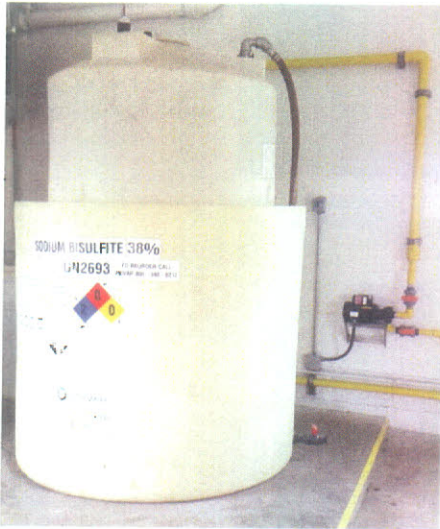
SBS pumps and back-up containment.
