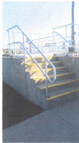
High visible paint for safety.
